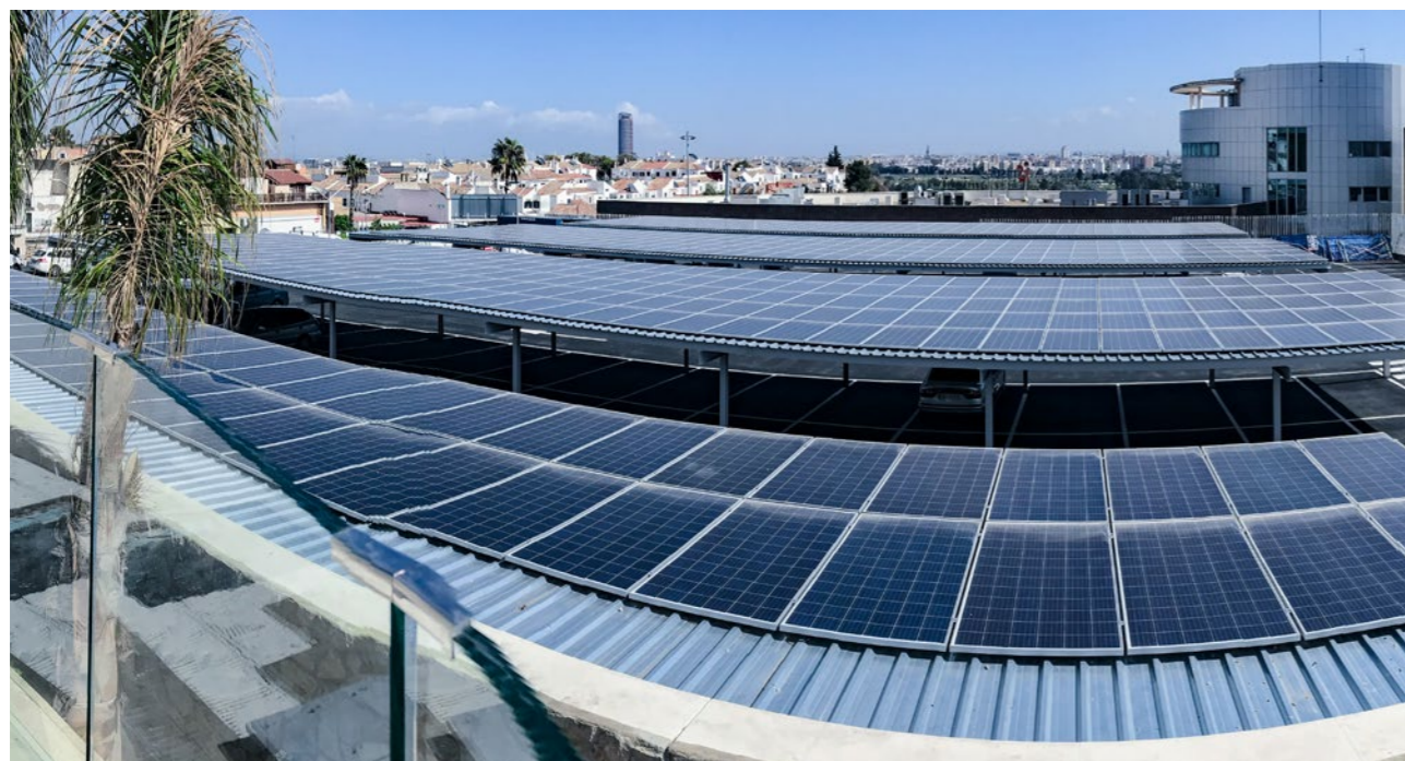
Photovoltaikanlage Gran Casino in Sevilla
